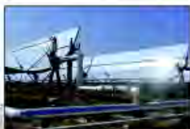
Heat transfer fluid in this solar thermal plant operates at a punishing 400°C
