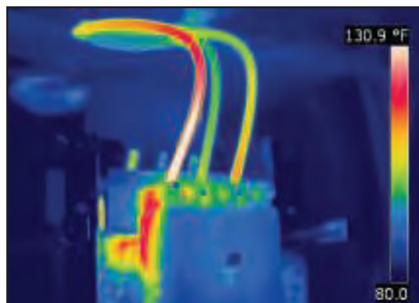
FIGURE 4. Infrared thermographic inspections of electrical auxiliary equipment related to plant machinery can reveal “hot spots” that are commonly found in equipment prior to failure. Loose connections, faulty components, overloaded parts and high friction are some of common problems that can be found during a thermographic scan. All “exceptions” should be properly documented with thermal and digital images that can be used in the condition monitoring
